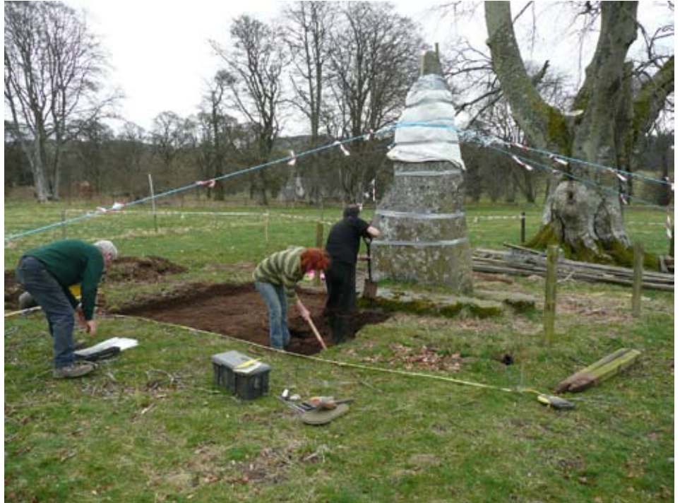
John Bel Stone: Carefully digging out the warren of rabbit burrows to stabilise the stone.
