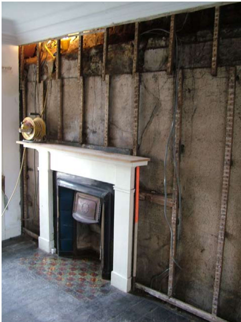
Two early plaster surfaces (one on top of the other) revealed after 19th-century laths were removed. The 17th-century stone fire surround was just visible behind the later mantelpiece.
